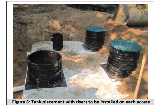
Figure 6: Tank placement with risers to be installed on each access port and brought to grade.
